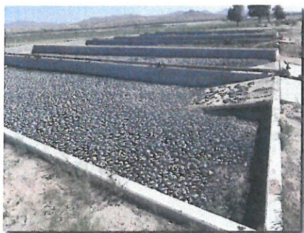
Sludge Drying Beds
