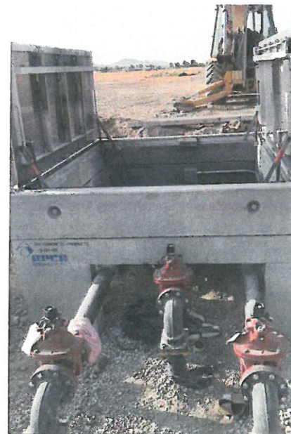
Secondary Irrigation manifold
