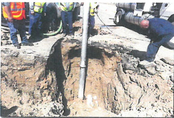
Force main break in 2016. This force main was replaced in 2019 at a cost of $329,760.
